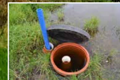
Control well where the water level can be raised and lowered.
